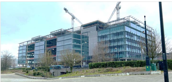
WSP used iterative design to lower the amount of concrete needed by 16,000 tons, save significant material costs, and greatly reduce carbon emissions.
